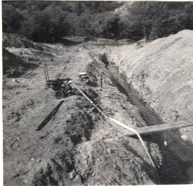
Pump in place.
